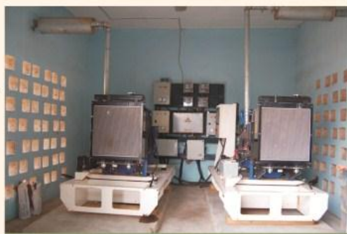
Newly acquired generators for pumping water
