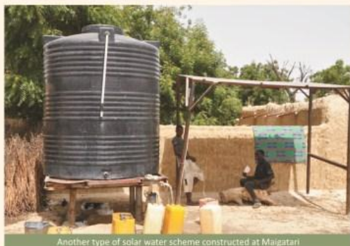
Another type of solar water scheme constructed at Maigatari
